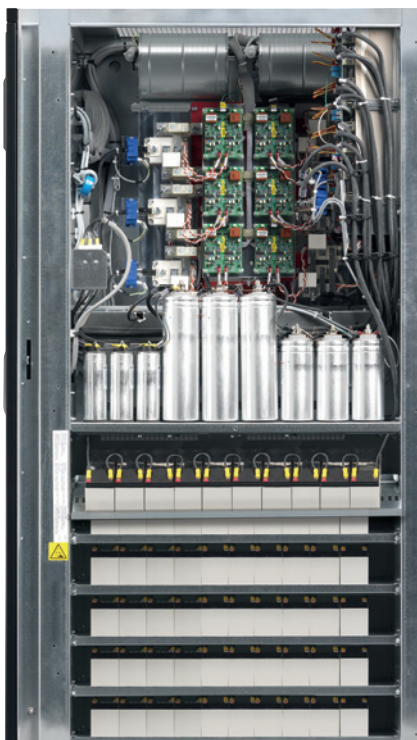
INTERNAL BATTERY FIXTURES
